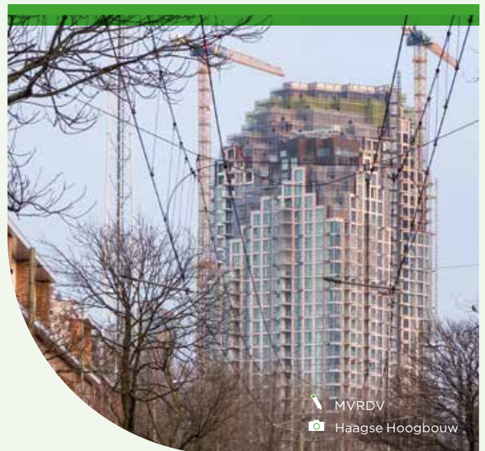
Grotius residential towers Closed cladding installed at the crown of the buildings - The Hague, the Netherlands
