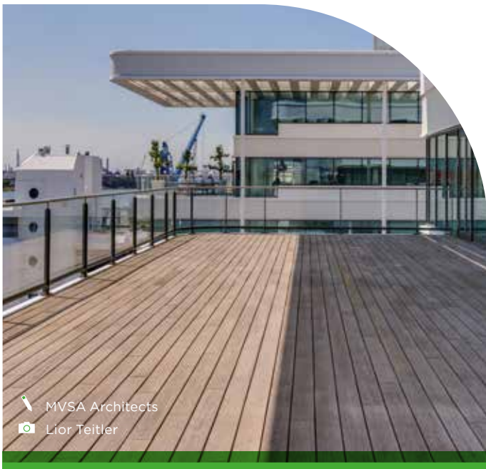
Jumbo Head office Photo taken 5 years after installation (2.500 m 2 ) Schiedam, The Netherlands
